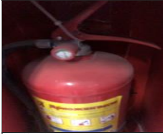
Photo of fire safety equipment IMG_3997.jpg
